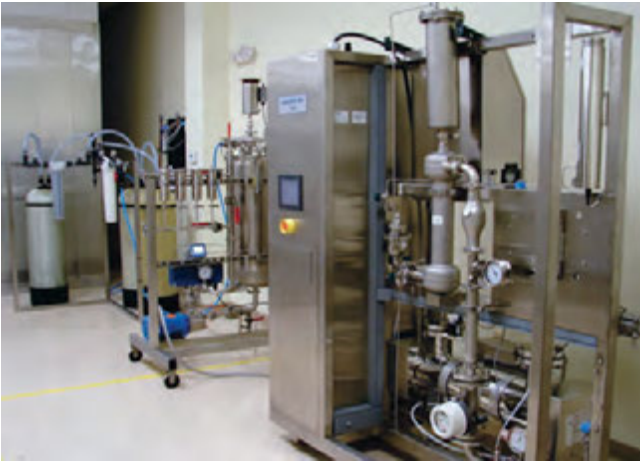
Figure 1. The full experimental test skid and water system used in this study.
