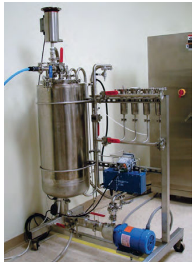
Figure 2. Close-up of the storage tank and coupon sampling system.
