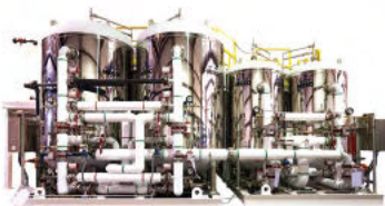
Carbon Filters & Softeners
