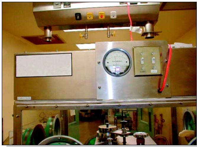
Figure 4. Press isolator magnehelic gauge.
