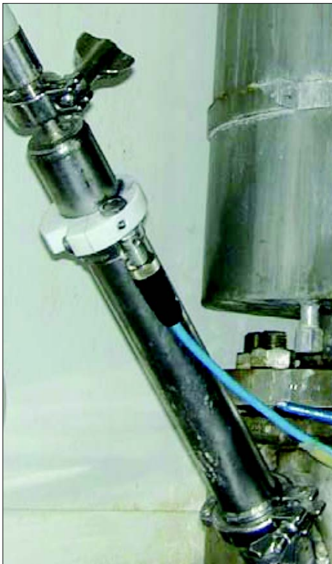
Figure 11. Extending spray unit which extends when the cleaning solution pressure is high enough.
