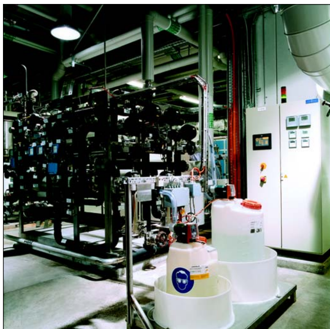
Figure 7. Operating and control panel, Dosing group for caustic soda and sodium bi-sulfite, Double-stage reverse osmosis (extensible).
