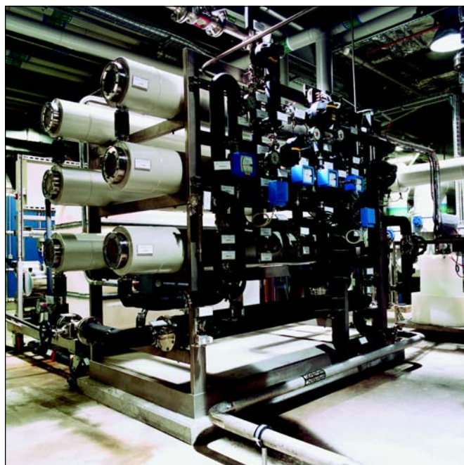
Figure 4. Double-stage reverse osmosis (extensible).
